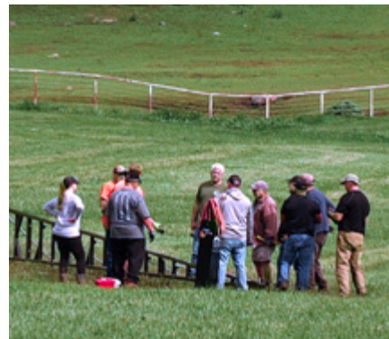
The volunteers gather, ready to begin the task of assembling the wall. (Photo by How Miller)
