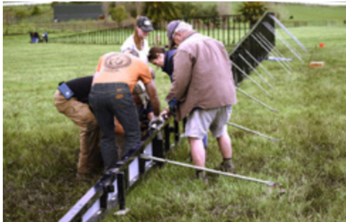
Mounting the panels starts from both ends, finishing in the middle. (Photo by How Miller)
